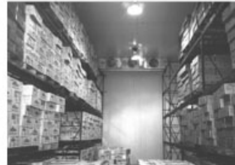
Hipac/Hanshell Inniss Bridgetown, Barbados Food Processing/ Cold Storage Frozen Food Storage -25°C
